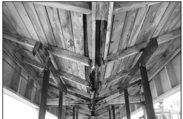
Fullerton Heritage is seeking ways to repair the loading dock roof to arrest the deterioration, restoring this element of the National Registered Fullerton Depot.
